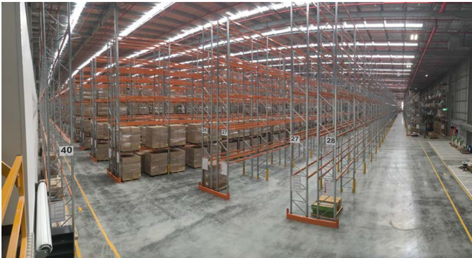
In-rack fire sprinklers installed in 1/4 of warehouse.
